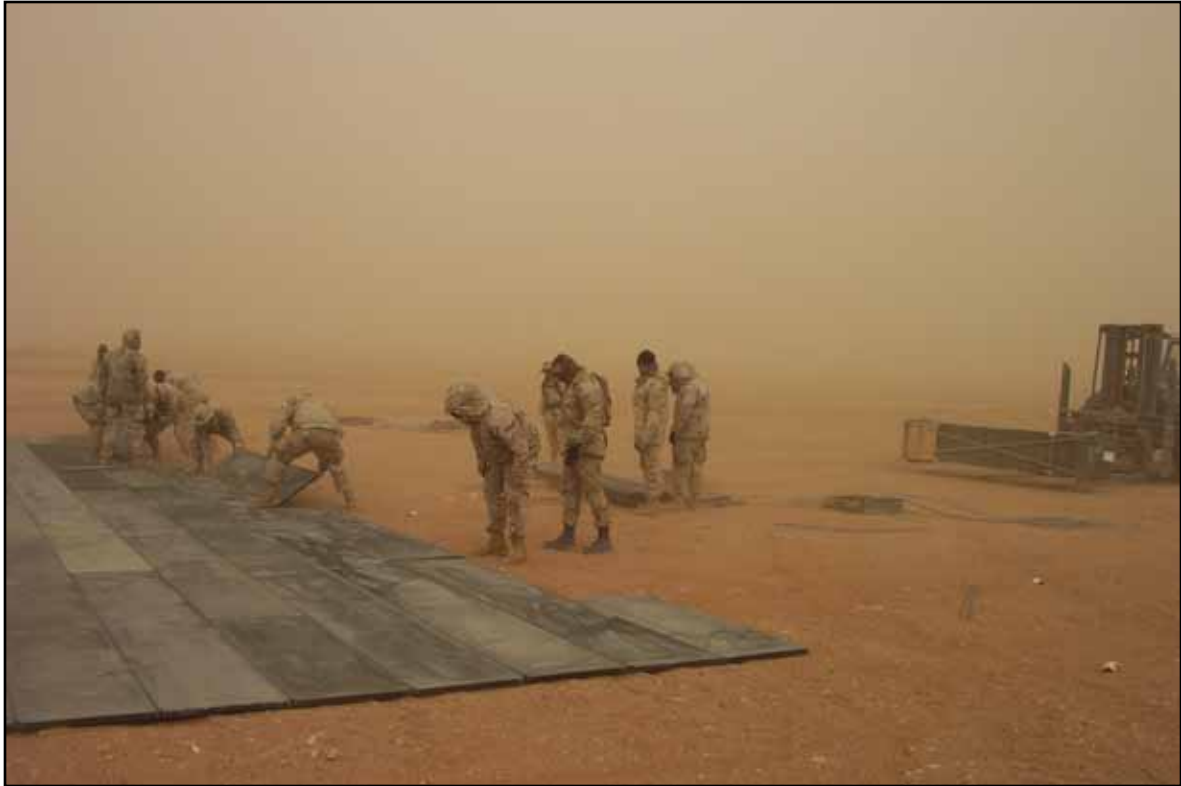
Engineers lay AM-2 matting in a dust storm at a base in preparation for Operation Iraqi Freedom combat operations.
