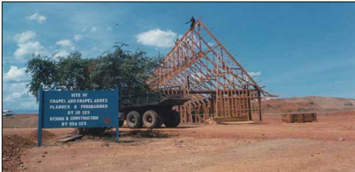
(below) A chapel under construction by the 554th RED HORSE Squadron at Phan Rang AB, South Vietnam.
