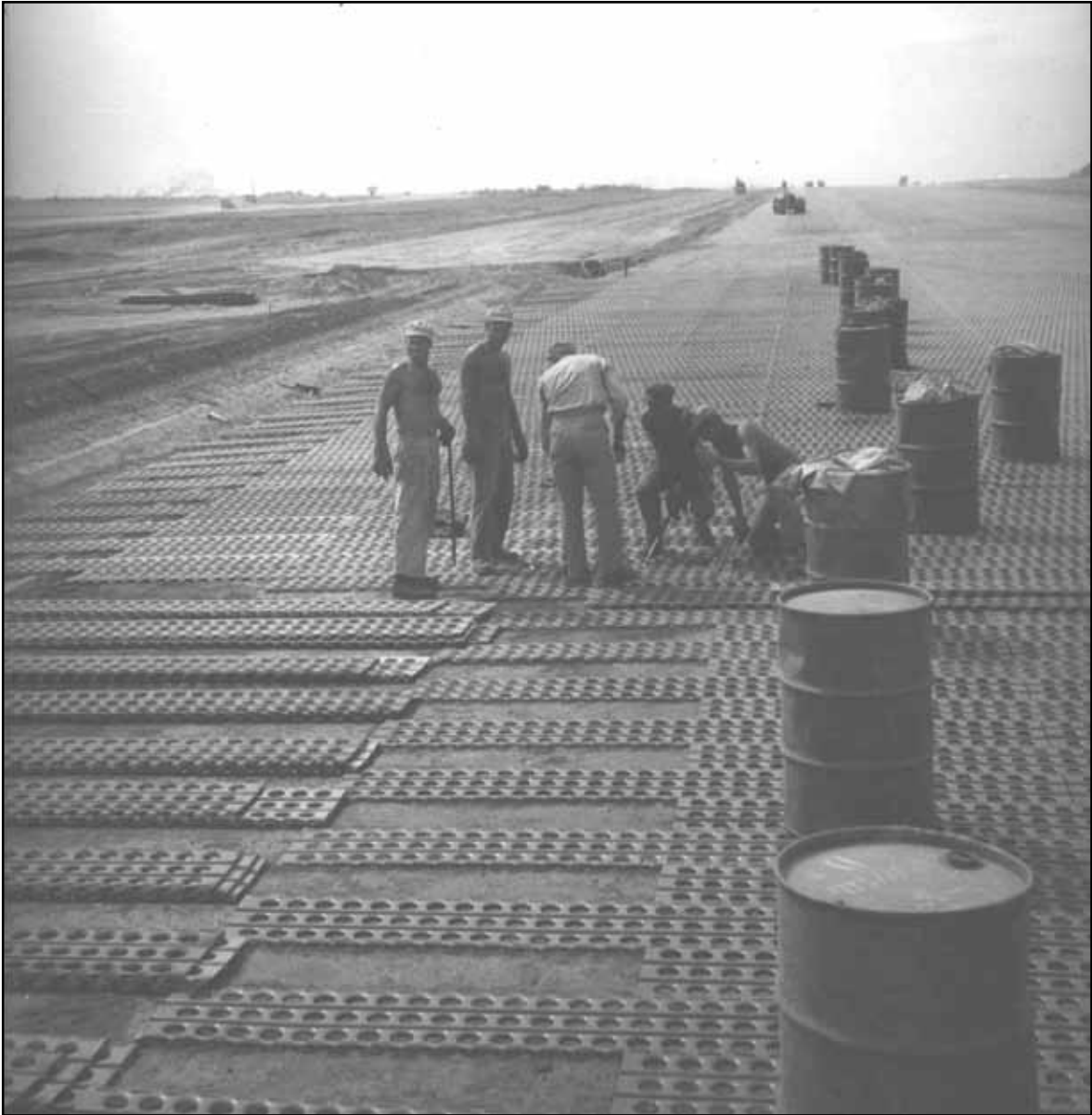
Engineers of the 1913th Engineer Aviation Battalion lay steel matting at Clark Field, Luzon, Philippine Islands.
