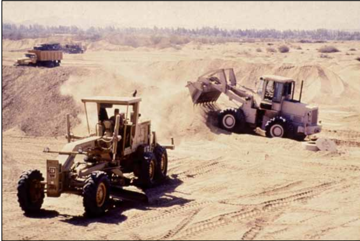
Air Force heavy equipment operators at work building a weapon storage area at a Gulf War site.
