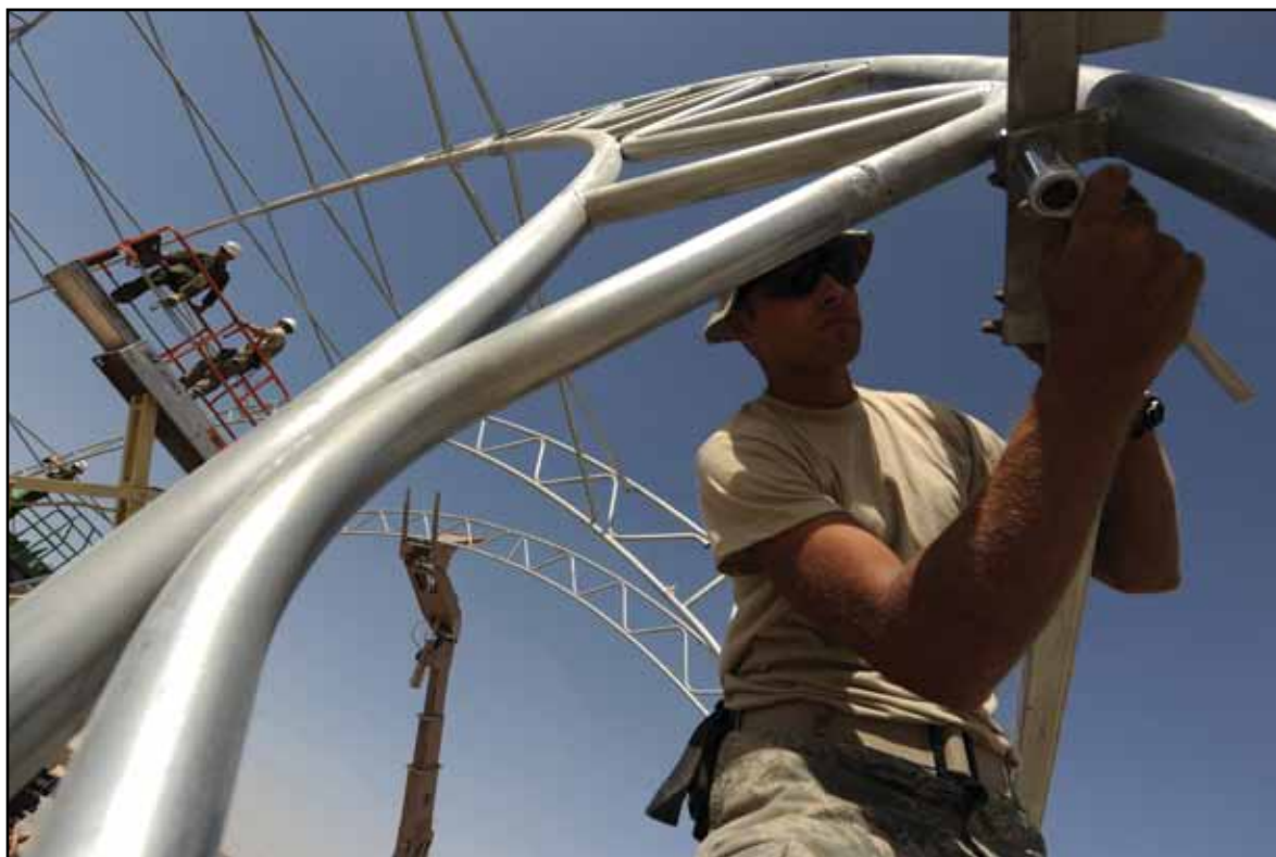
SrA Jonathan Carmona, a structural journeyman assigned to the 777th Expeditionary Prime BEEF Squadron, secures square tubing to a metal frame at Kandahar Airfield, Afghanistan.
