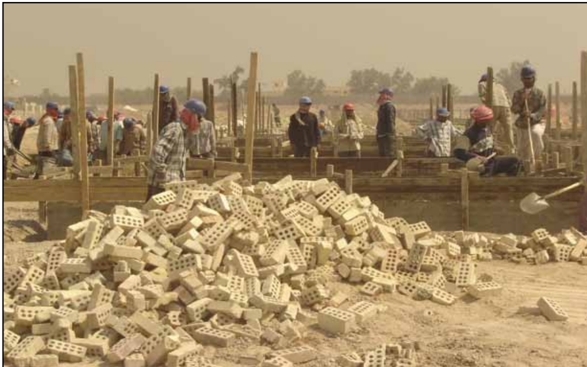
Iraqis work to complete an enlisted barracks at an Iraqi military base.
