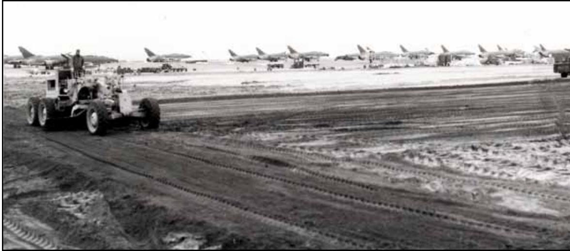
Members of the 820th RED HORSE Squadron level a site in preparation for the construction of a maintenance apron at Tuy Hoa.
