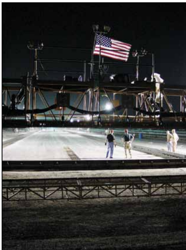
Members of the 820th RED HORSE Squadron use a paving machine at Al Dhafra acquired through AFCAP.
