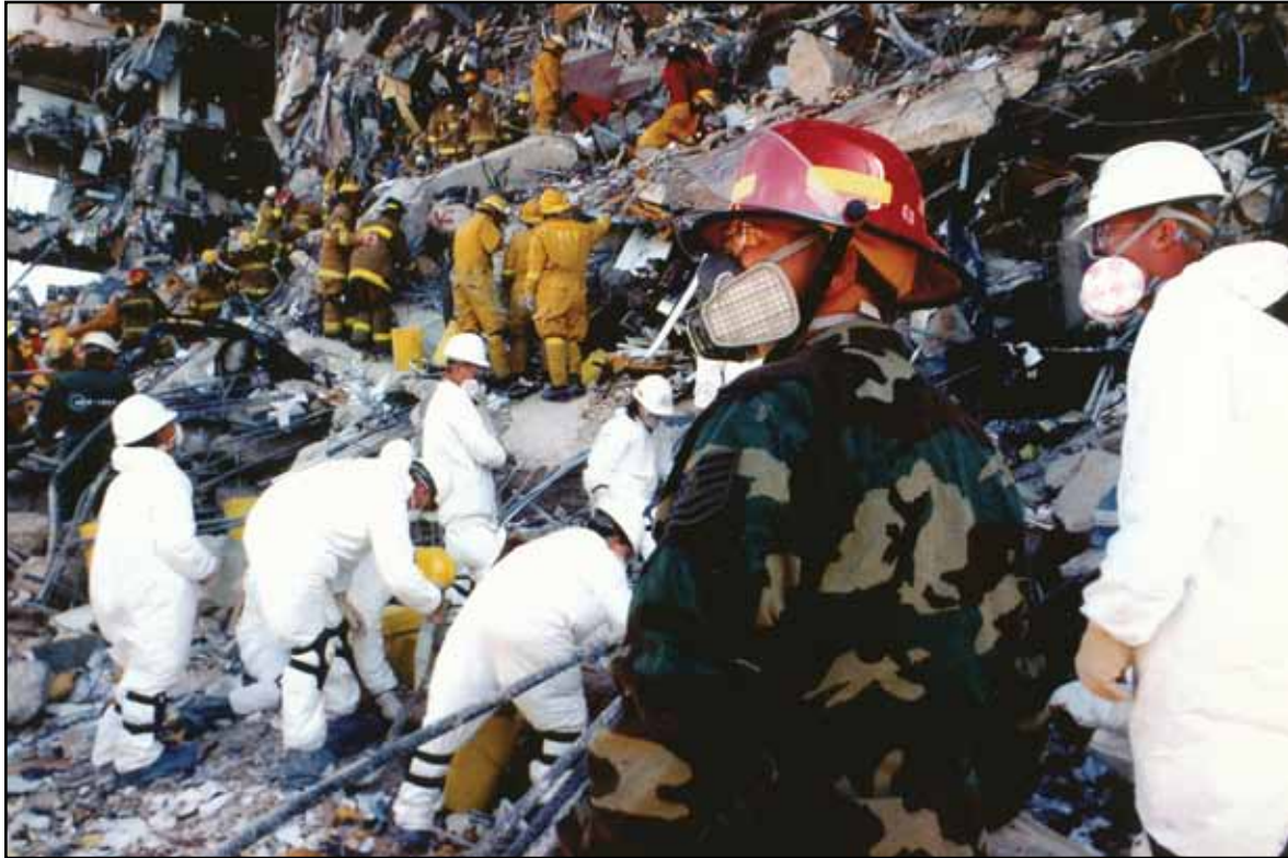
A firefighter from Tinker AFB, Oklahoma, surveys the damage at the Alfred P. Murrah Federal Building in downtown Oklahoma City.
