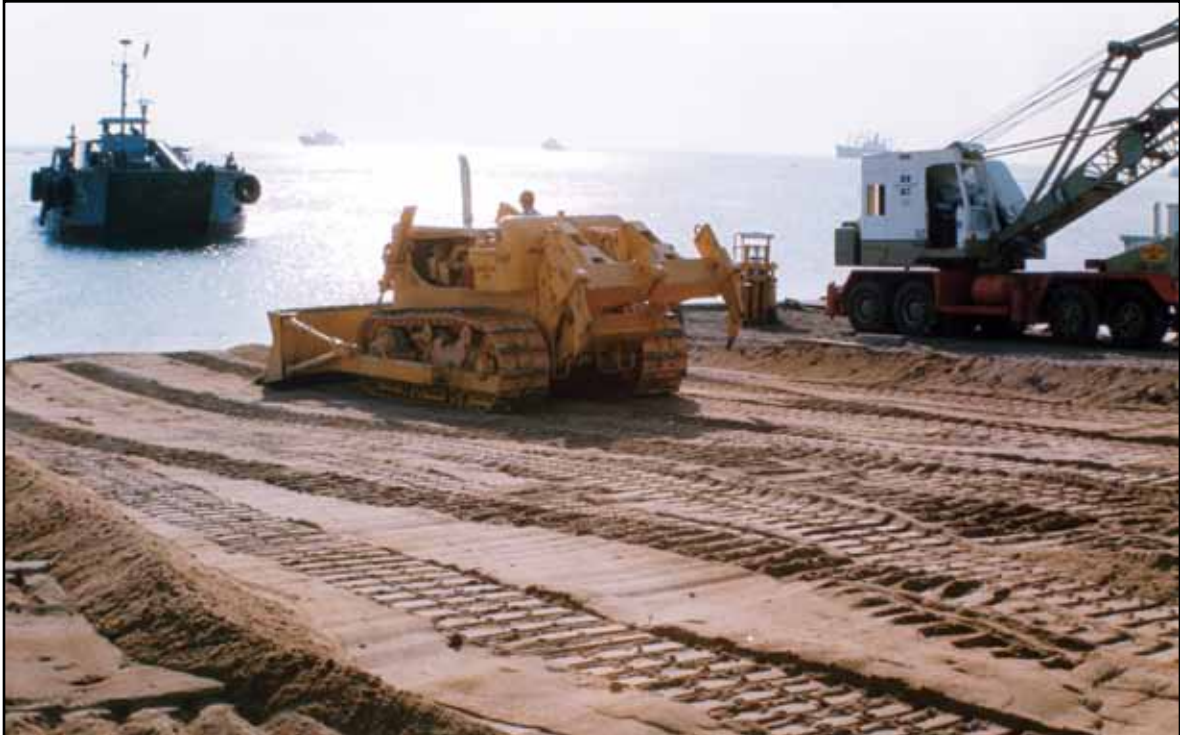
A bulldozer levels the beach as a landing craft approaches bringing in equipment and supplies for the buildup of Tuy Hoa.
