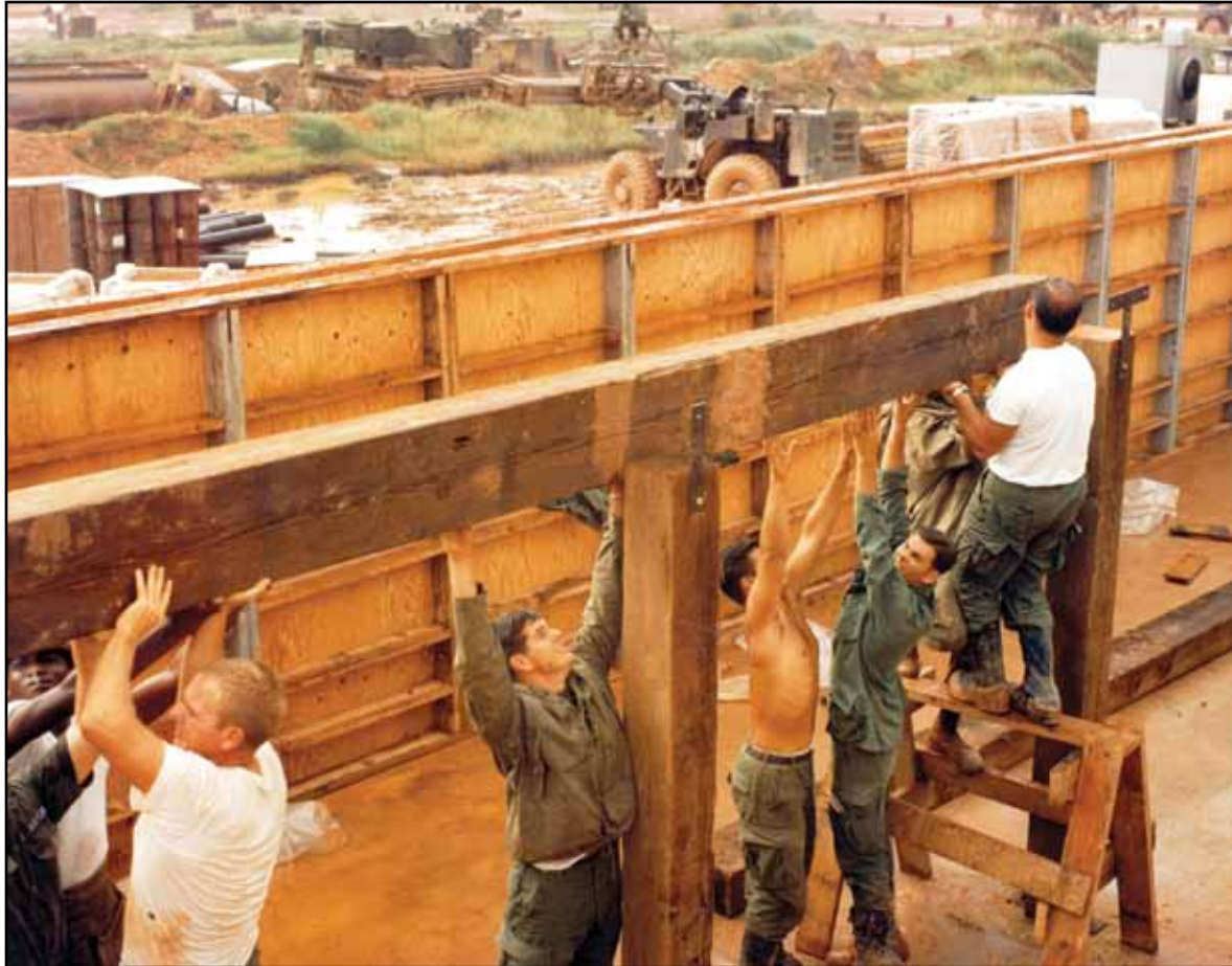
Members of the 820th RED HORSE Squadron build a bunker at Dong Ha, South Vietnam. The person in the middle of the photo wearing a jacket is Airman 1st Class Larry R. Daniels. He later became the first Chief of Enlisted Matters for Civil Engineering in 1989.
