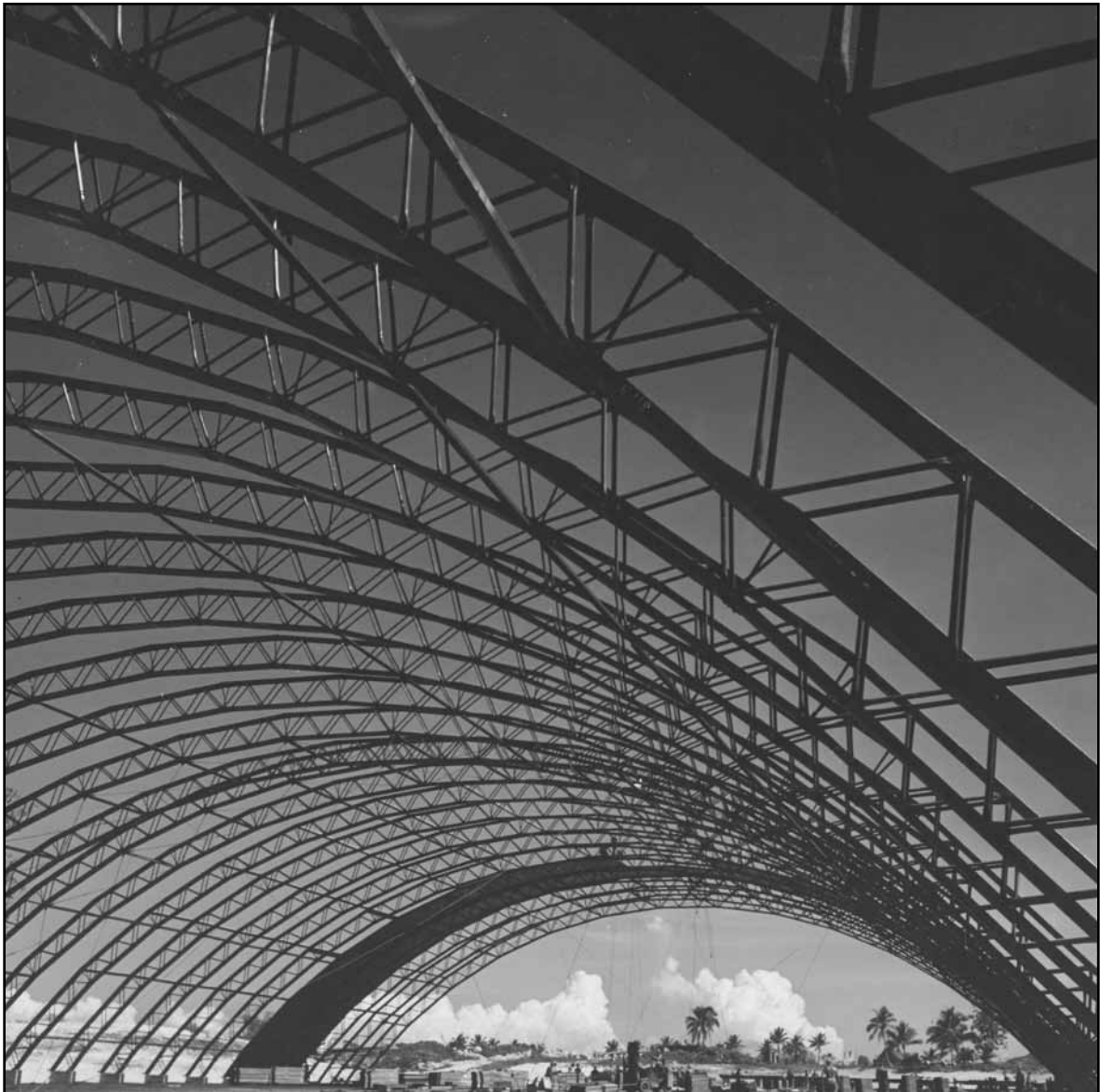
A hangar under construction at a 7th Air Force base in the Pacific.
