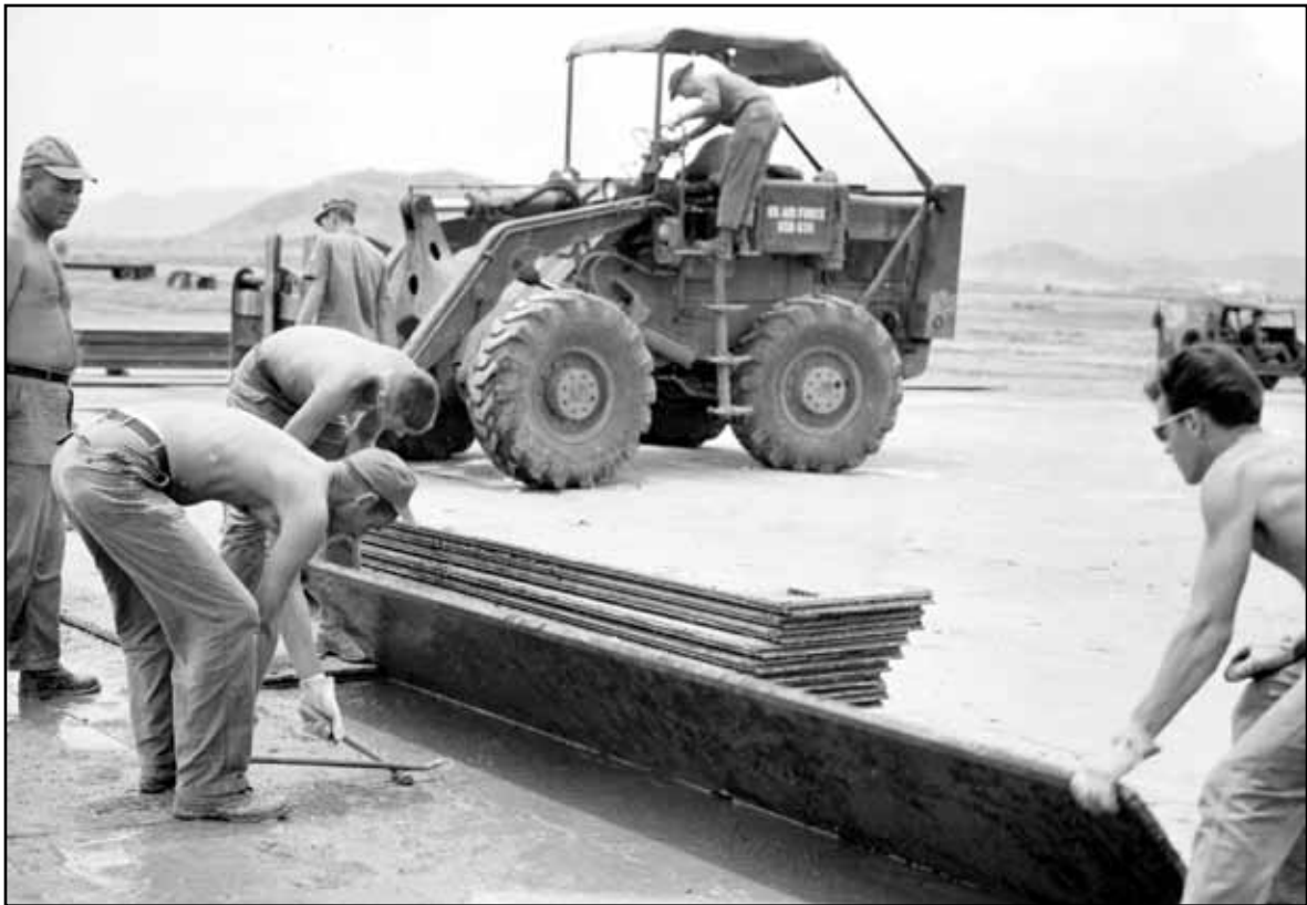
(above) 554th RED HORSE personnel take up AM-2 matting to expose the damaged base to begin repairs at Phan Rang AB, South Vietnam.
