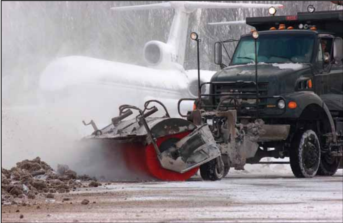
Members of the 376 Expeditionary Civil Engineer Squadron clear snow and ice from runways for aircraft at Ganci Air Base, Manas International Airport, Kyrgyzstan.
