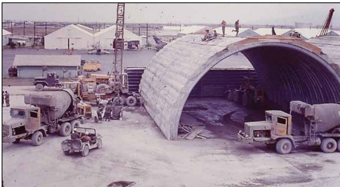
819th RED HORSE Squadron constructs hardened aircraft shelters at Da Nang AB, South Vietnam. (Courtesy of Col. Allen Sailer.)
