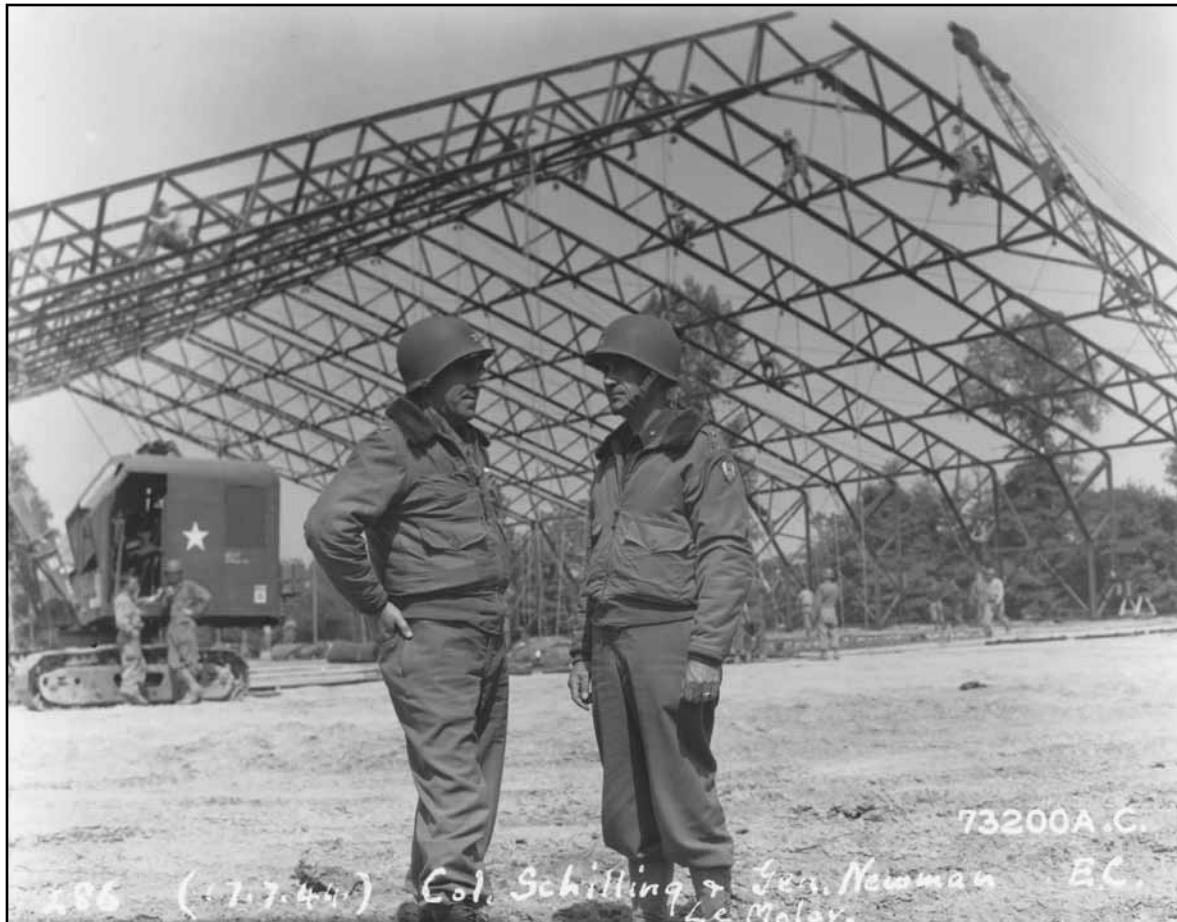
Brig. Gen. James B. Newman (right), Commander, IX Engineer Command, and Col. Karl B. Schilling, Commander, 1st Engineer Aviation Brigade, tour an airfield near LeMole, France, where a Butler Building is under construction.
