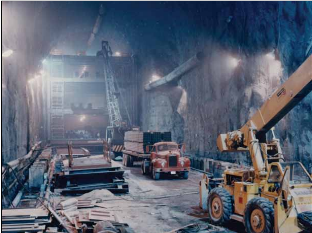
Construction inside one of the chambers of the NORAD Cheyenne Mountain Complex.
