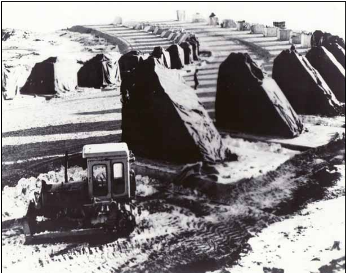
Hot air inside an air-supported tent protects construction workers from falling temperatures at a base of the Ballistic Missile Early Warning System.
