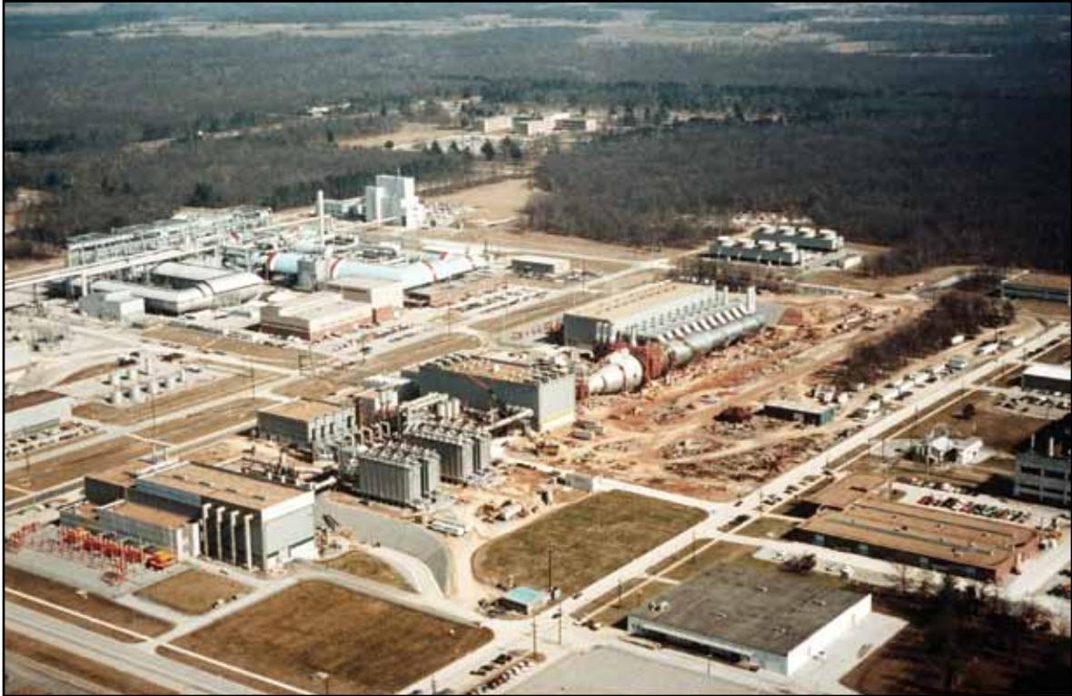
An aerial view (looking west) of the Aeropropulsion System Test Facility (ASTF) under construction at the Arnold Engineering and Development Center, 1983.
