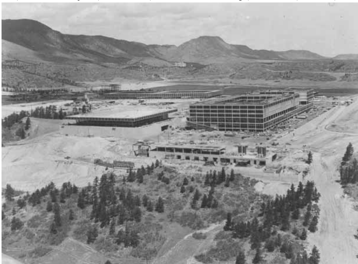
U.S. Air Force Academy under construction with the Colorado Rockies as a dramatic backdrop.
