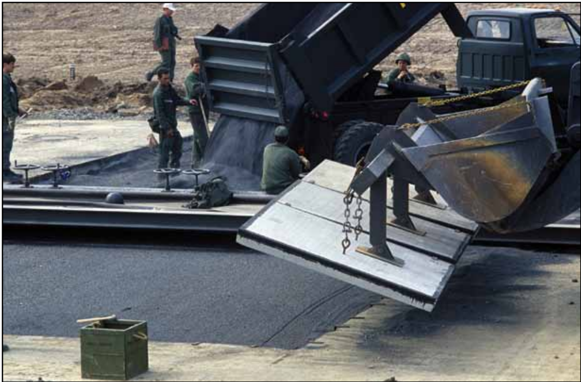
Rapid Runway Repair in progress at Spangdahlem AB, West Germany, during Salty Demo, 1985.
