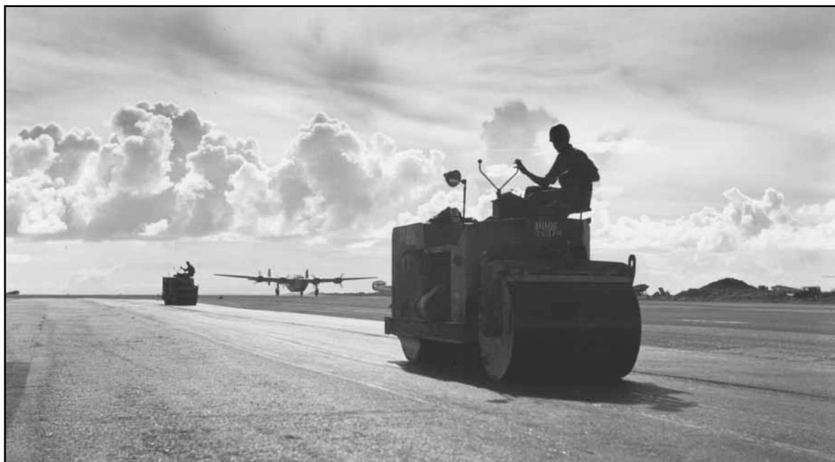
Rollers smooth a runway surface as a B-24 Liberator lands following a long, overwater strike. This black-topped airstrip gave an all-weather capability for the aircraft in the Bonin Islands.
