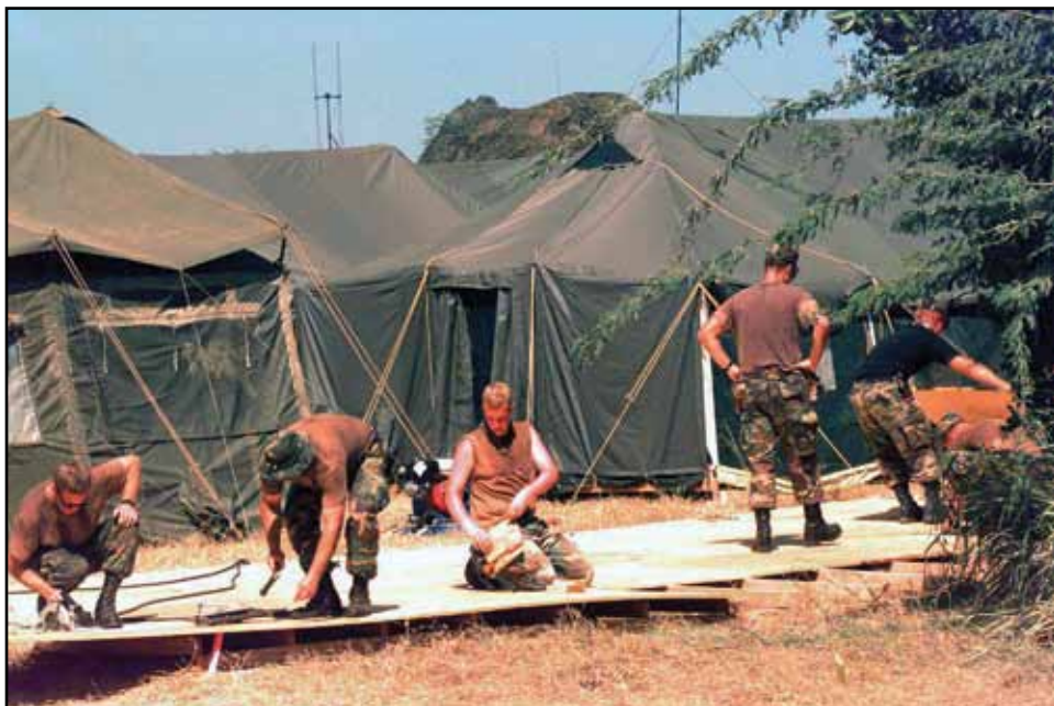
Carpenters from the 820th RED HORSE Squadron, Nellis AFB, Nevada, put together a hard wood floor for a future tent location in Port au Prince, Haiti in support of Operation UPHOLD DEMOCRACY, 1994.
