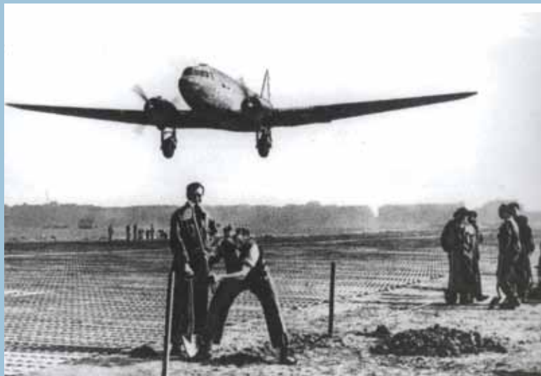
While the new runways were built, the old ones had to be repaired. Workers repair the runway at Tempelhof using hand tools.
