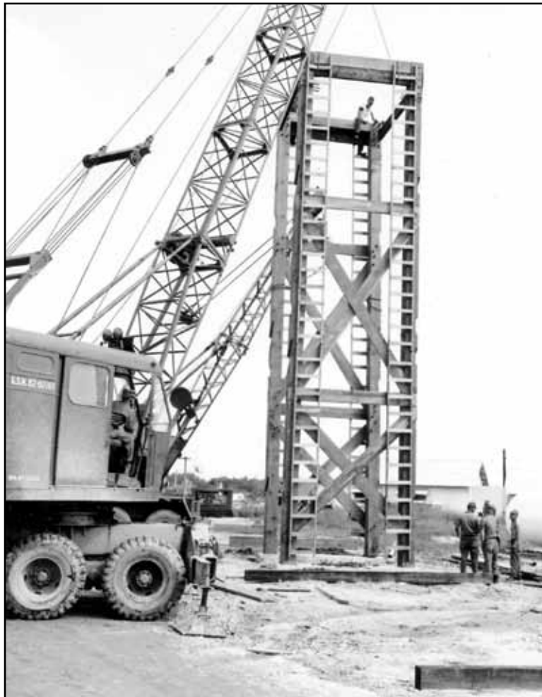
A Prime BEEF team constructs a water tower at Da Nang AB, November 1966.
