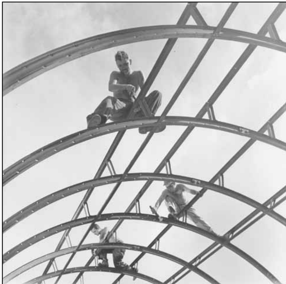
Aviation engineers construct steel frame for the roof on a Quonset hut on Saipan,
