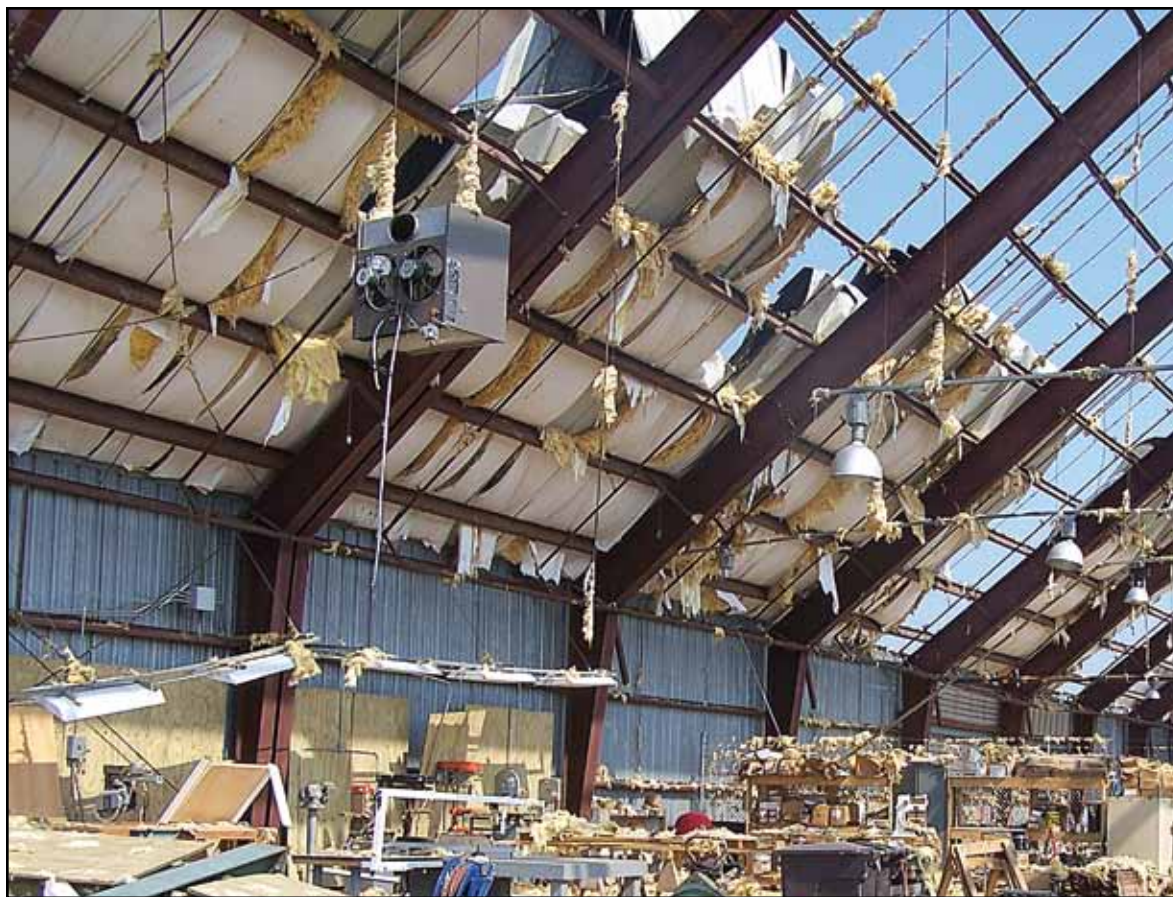
Hurricane Katrina did extensive damage to Building 4422 at Keesler AFB, Mississippi.
