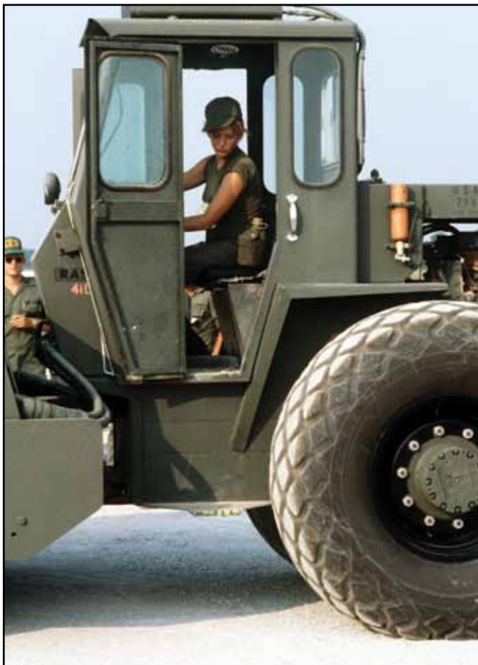
A1C Susan Miller operates a 10-ton roller used to compact crushed limestone during a simulated runway attack Prime BEEF exercise at North Field, 1980.
