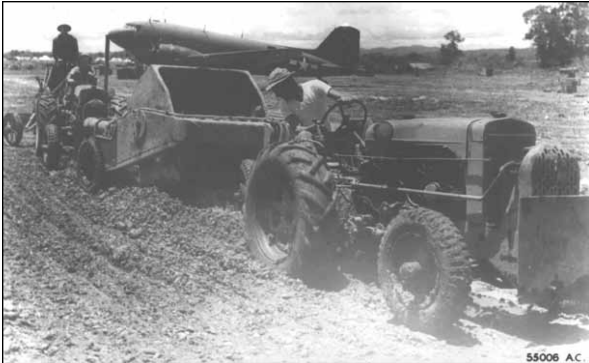
Airborne aviation engineers work on the Myitkyina airstrip for use by 10th Air Force pilots.
