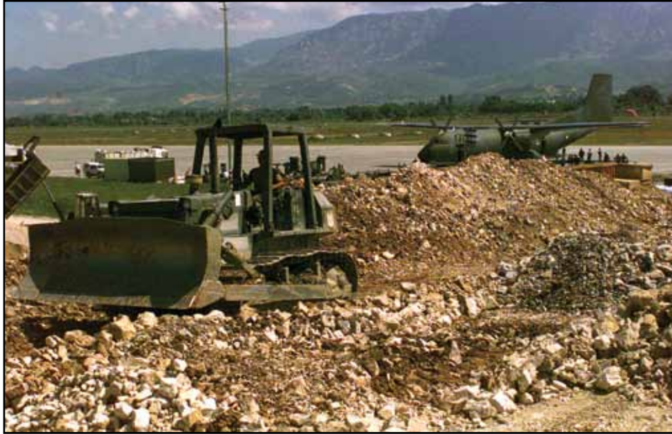
Engineers from the 823d RED HORSE Squadron move dirt at Rinas Airport, Tirana, Albania, during Operation ALLIED FORCE, 1999.
