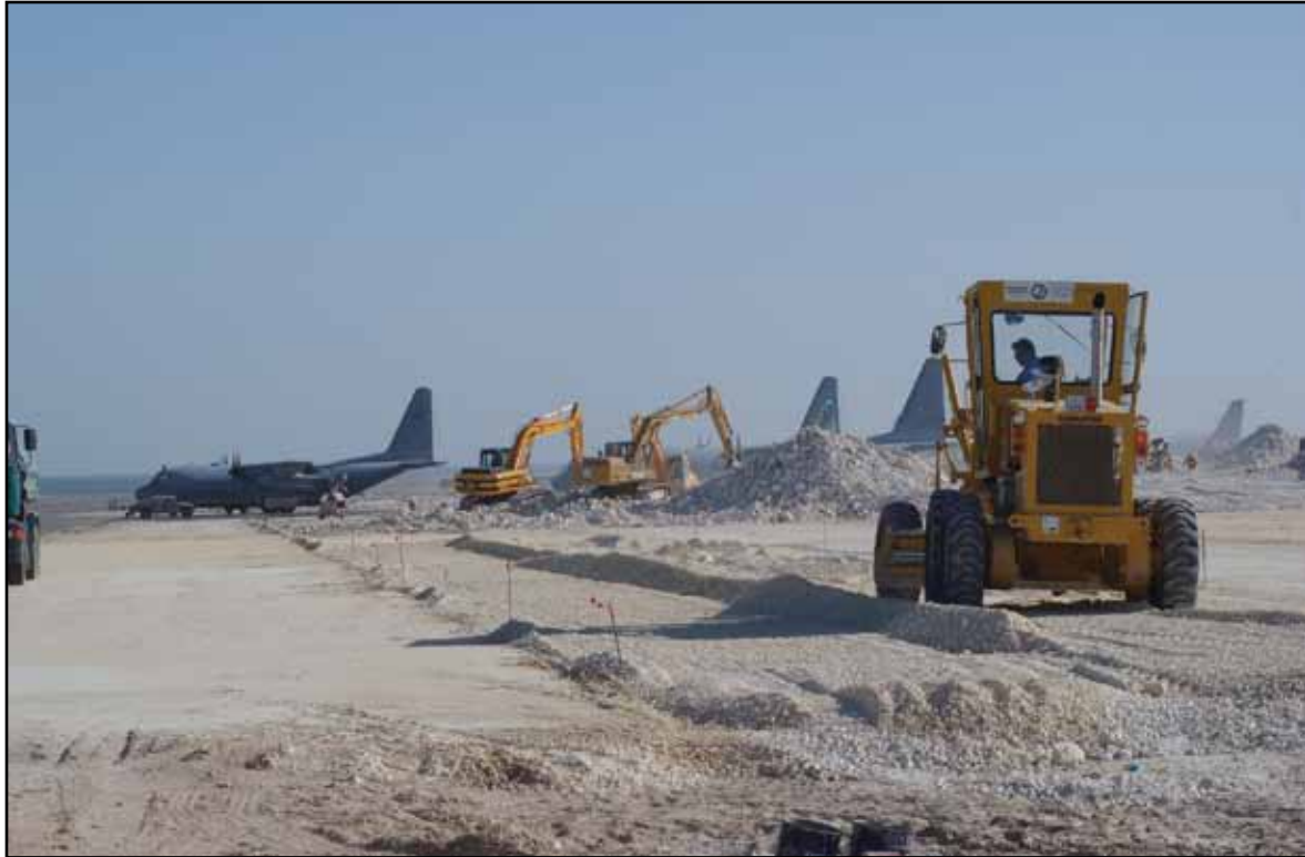
Civil engineers from Travis AFB, California, support the buildup of forces at Shaikh Isa AB, Bahrain.
