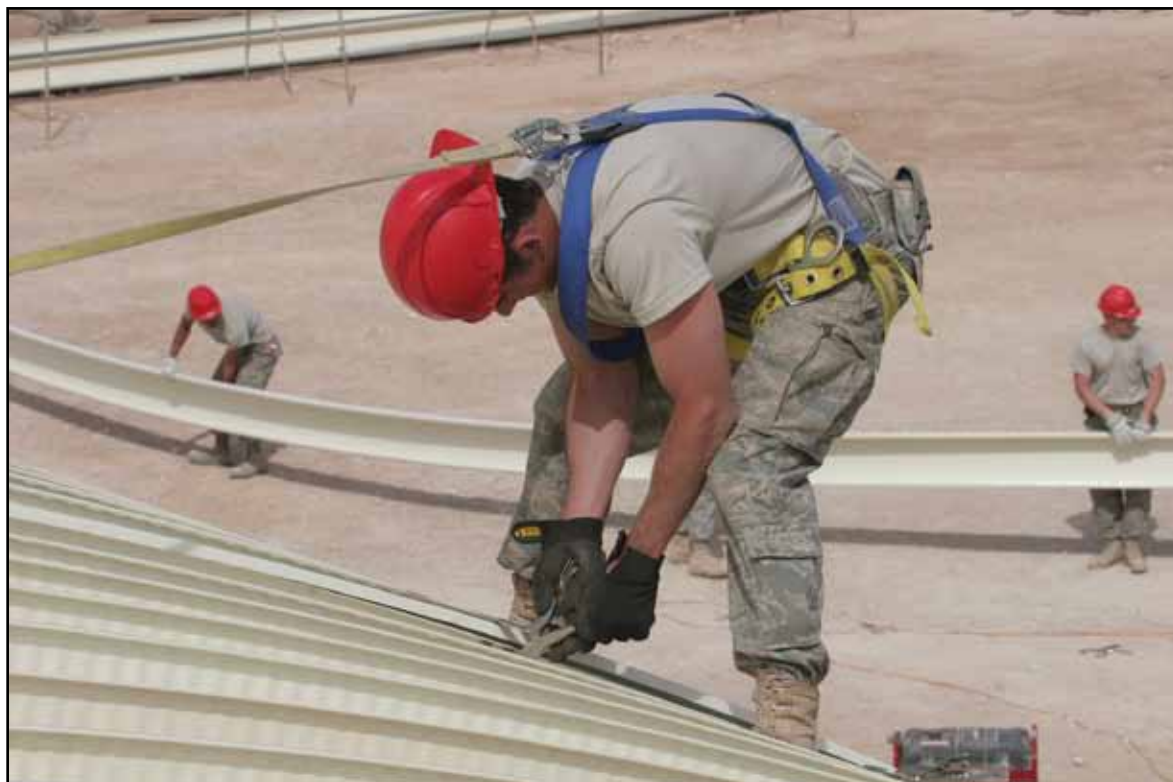
U.S. Air Force SrA Franklin Travis Kee, with the 557th Expeditionary RED HORSE Squadron, clamps two panels together while building a new supply warehouse at Camp Ripper, Iraq.
