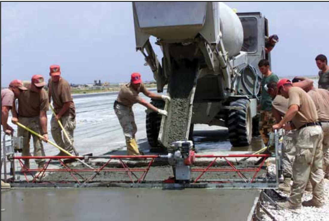
The 200 RED HORSE Squadron and 201 RED HORSE Flight make repairs to the runway at Bagram AB, Afghanistan in 2002.
