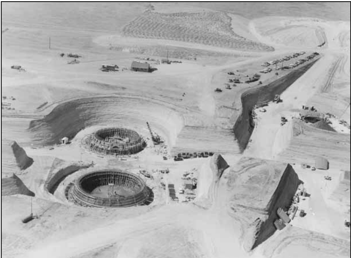
This mammoth excavation near Denver, Colorado, will soon be an almost invulnerable underground launch site for the Air Force Titan ICBM.
