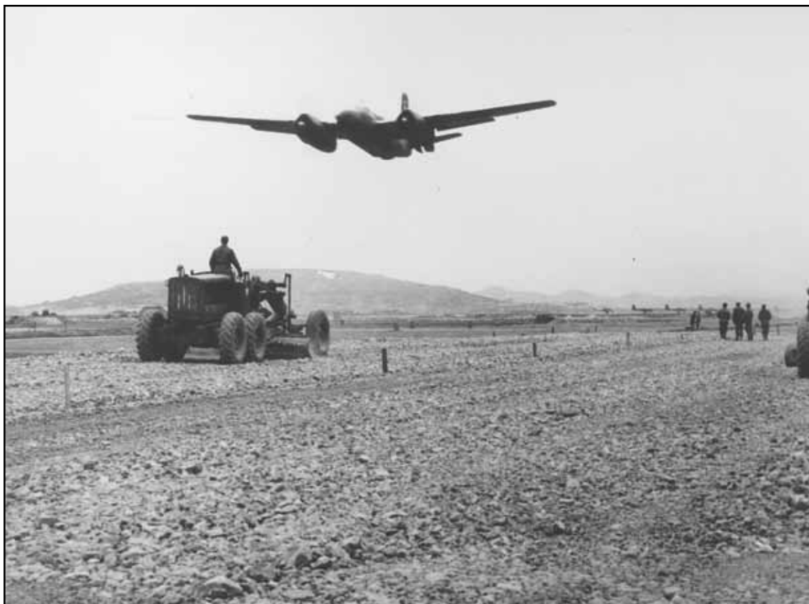
Members of the 808th Engineer Aviation Battalion transform a rice paddy into an airstrip in Korea.
