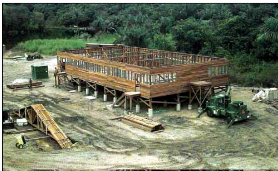
Members of the 820th RED HORSE Squadron, Nellis Air Force Base, Nevada, work on rebuilding the Malali District schoolhouse as part of New Horizons-Guyana 1997.
