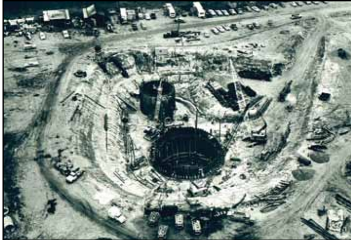
An Atlas F underground silo under construction at Plattsburgh AFB, New York, ca. 1961.
