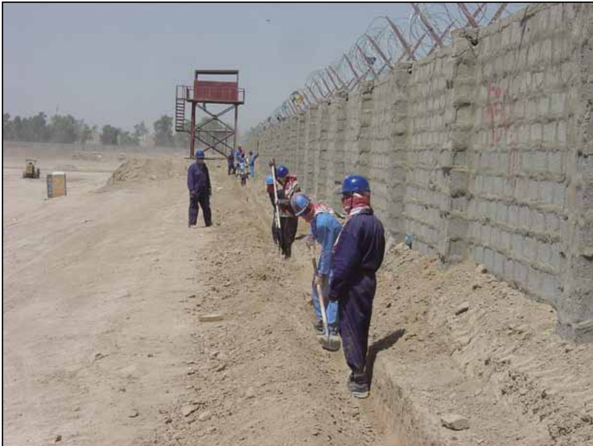
Iraqis complete trenching for perimeter lighting on a project completed under AFCEE's management.
