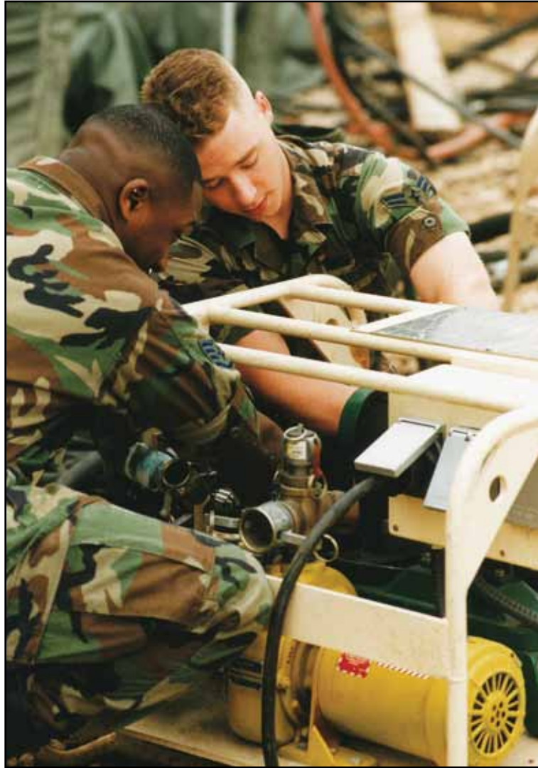
Members of the 52d CES, Spangdahlem AB, Germany, assemble a Harvest Eagle shower/wastewater distribution pump for a tent city at Aviano AB, Italy.
