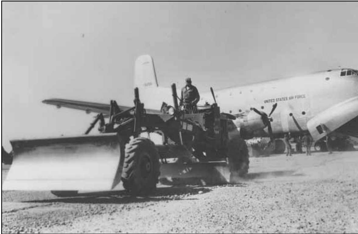
With an Air Force Douglas C-124 “Globemaster” unloading its cargo, an aviation engineer on a heavy road grader repairs a runway at a base in Korea.
