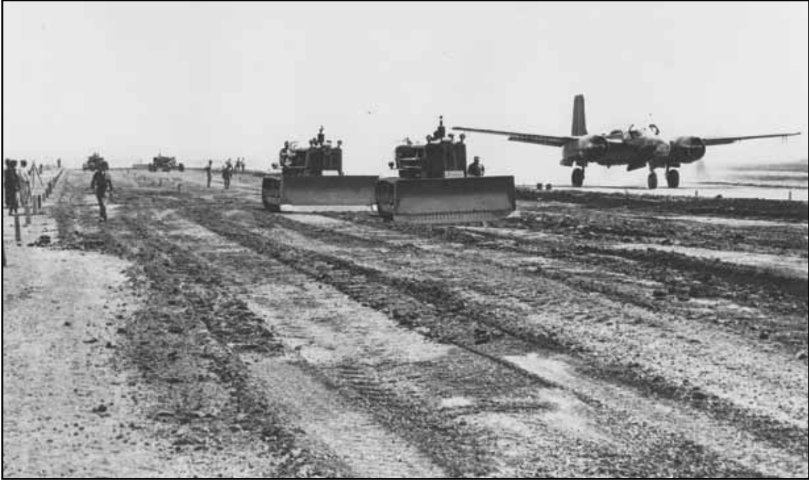
As a B-26 light bomber taxis alongside, members of the 808th Aviation Engineer Battalion continue grading an airstrip to support air operations.
