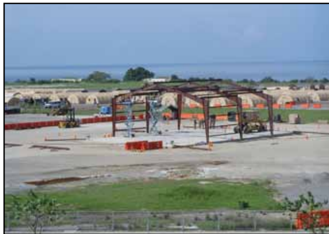
“Red Bull” civil engineers from the 474th Expeditionary Civil Engineer Squadron construct facilities at Camp Justice, Guantanamo Bay, Cuba.
