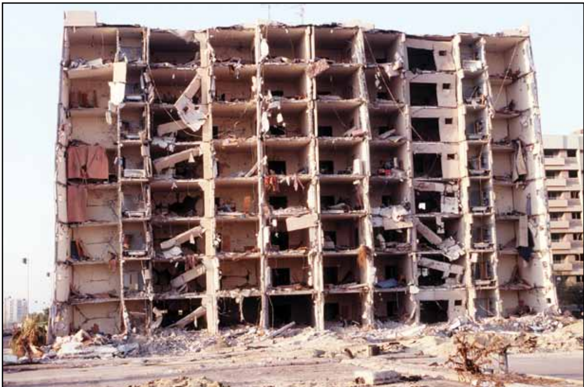
An overall view of the north side of the building that was severely bomb damaged in the Khobar Towers complex, 1996.
